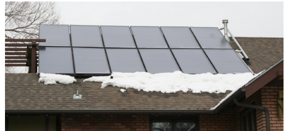
Solar panels visual impacts are minimized
